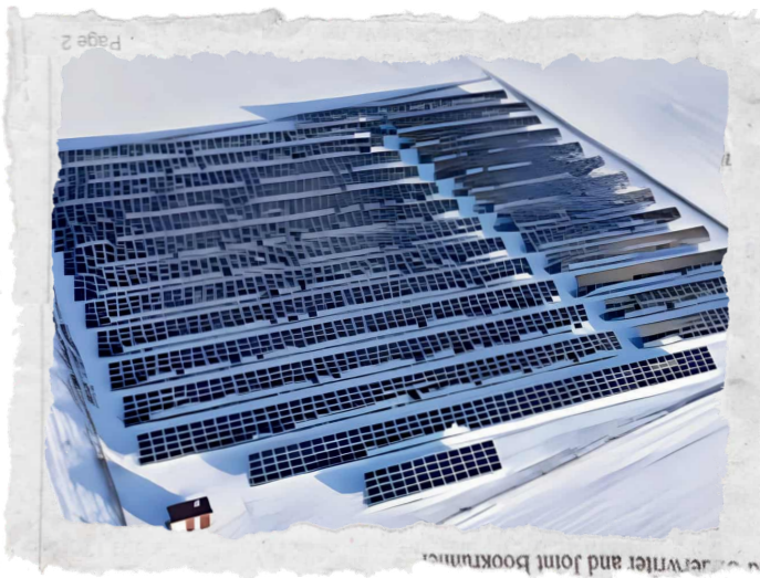
Figure 6: Solar farm in Finland
